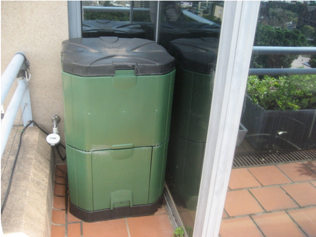
Aerobin compost bin on the balcony at Level 15, 179 Elizabeth Street.
